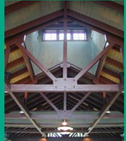
Exposed trusses and wood trim are painted brown with paneled surfaces in a natural cypress stain. The clerestoried cupola draws in natural light.
