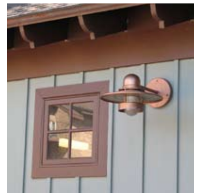
A detail shows board-and-batten siding, shaped rafter tails and a nautical light fixture.
